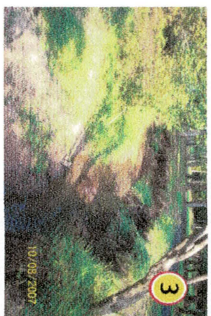
Whenever moving water meets a ripraped or steel pile there will always be erosion. - FEMA
